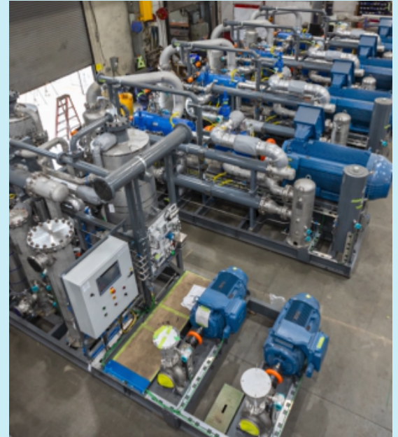
Compressors in the AdvanTec manufacturing facility in Chilliwack, BC
